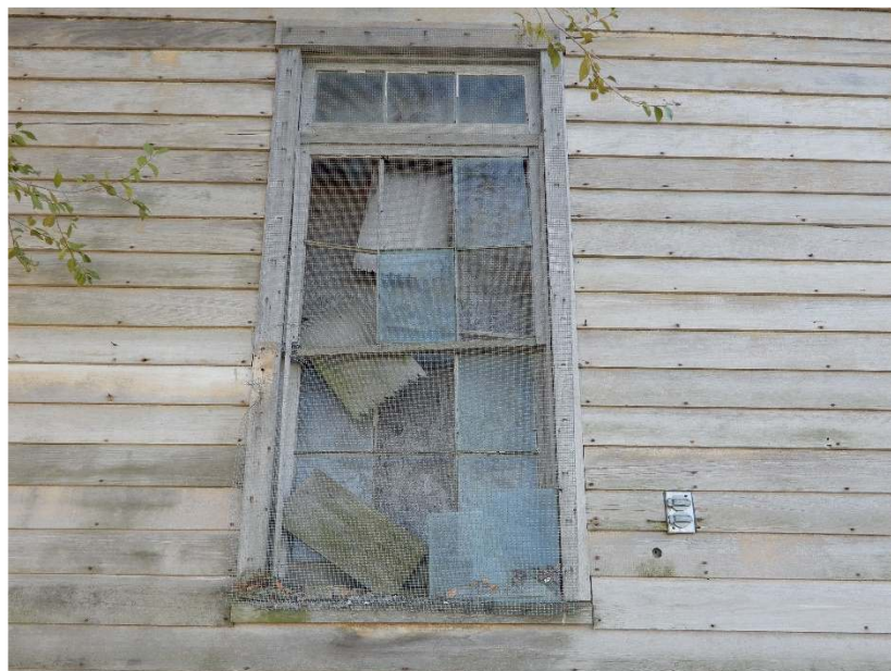
Detail of original window on north side of building showing distinctive three-light transom above 6/6 double-hung wood-sash window.
