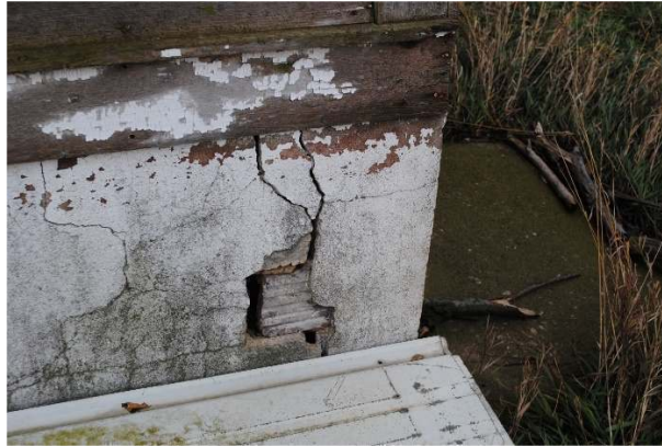
Prospect Hill School #3. Facing south. Detail of tile block foundation with concrete parging.
