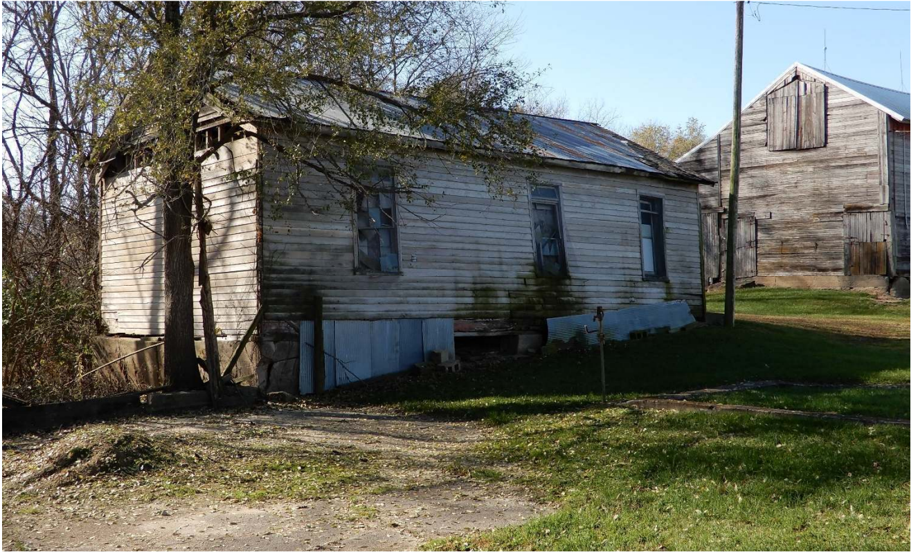
Looking SW at Cedar Center Schoolhouse showing north and rear sides of building.
