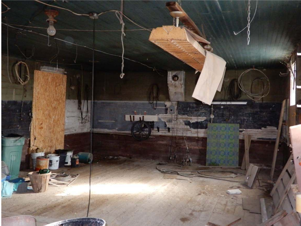
Interior of Cedar Center Schoolhouse looking ENE and showing remnant chalk boards, original hardwood floors, and beadboard ceiling.
