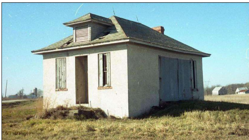
Figure 83. Circa 1996 photograph of the stuccoed White Prairie Schoolhouse as a closed and deteriorating building. Copy provided by Muscatine County HPC.
